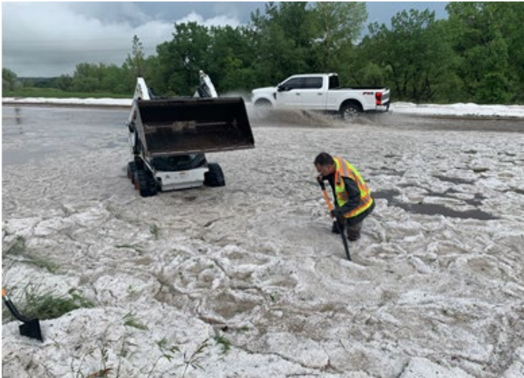
City workers unblocking drainage inlet clogged by hail during a June 2023 storm
