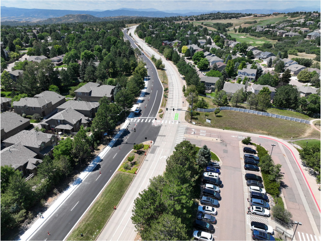
Eastbound Castle Pines Parkway, between Monarch Boulevard and Forest Park Drive, was reconstructed this summer.
