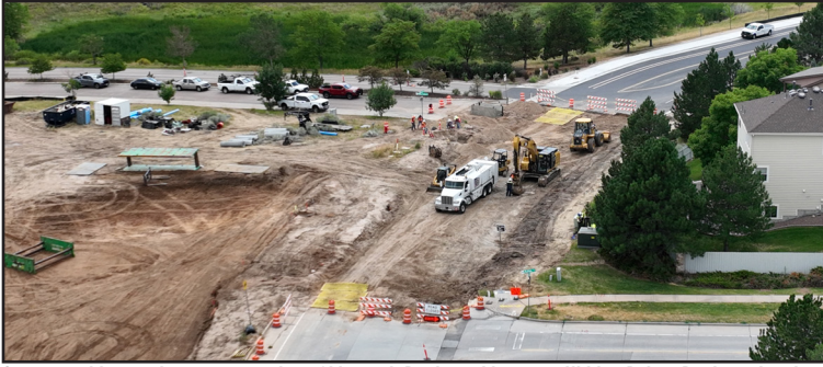
Crews working on the reconstruction of Monarch Boulevard between Hidden Pointe Boulevard and Buffalo Trail.
