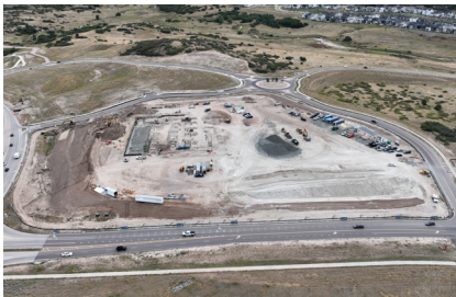
Site preparation and earthwork began early this summer for the Life Time facility at Castle Pines Parkway and Canyonside Boulevard.
