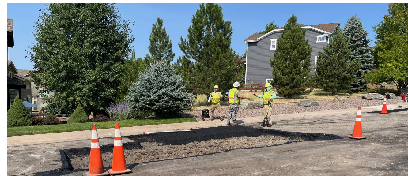
Over the summer and fall, crews will work on repairing neighborhood streets, curbs, and gutters to help extend the life of the City's roadway infrastructure as a part of the 2026 Pavement Maintenance Program.
