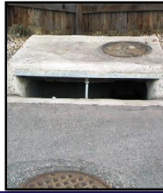
Denver No. 14 Curb Opening
