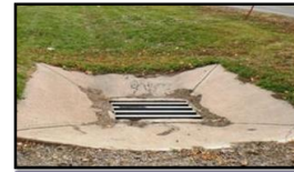
CDOT Type C Inlet in Depression
